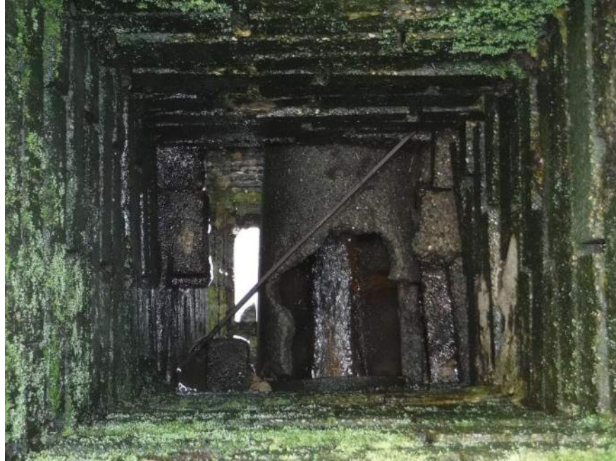
Image 5: Concrete pipe conveys flows through this CB
